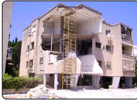
Haifa Katyusha Damaged House
